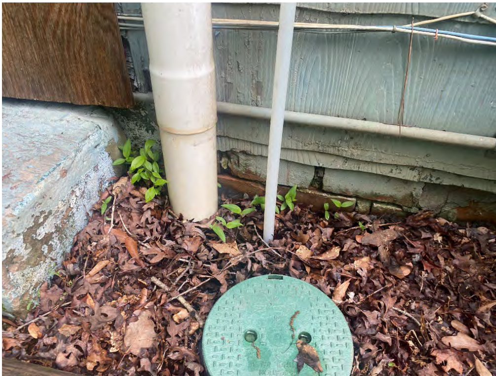
PHOTO 27: (View of Rear Façade, Rear Porch): Drainage system to be examined.
