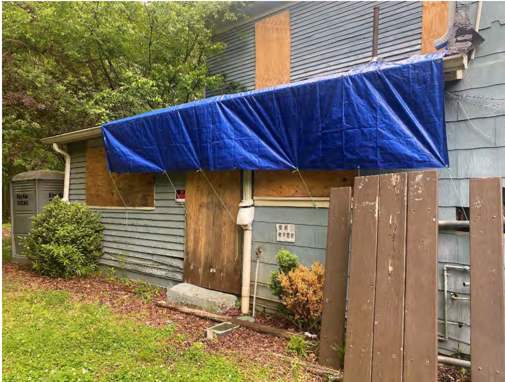
PHOTO 26: (View of Rear Façade): Rear Porch observed in poor condition, deemed unsafe.
