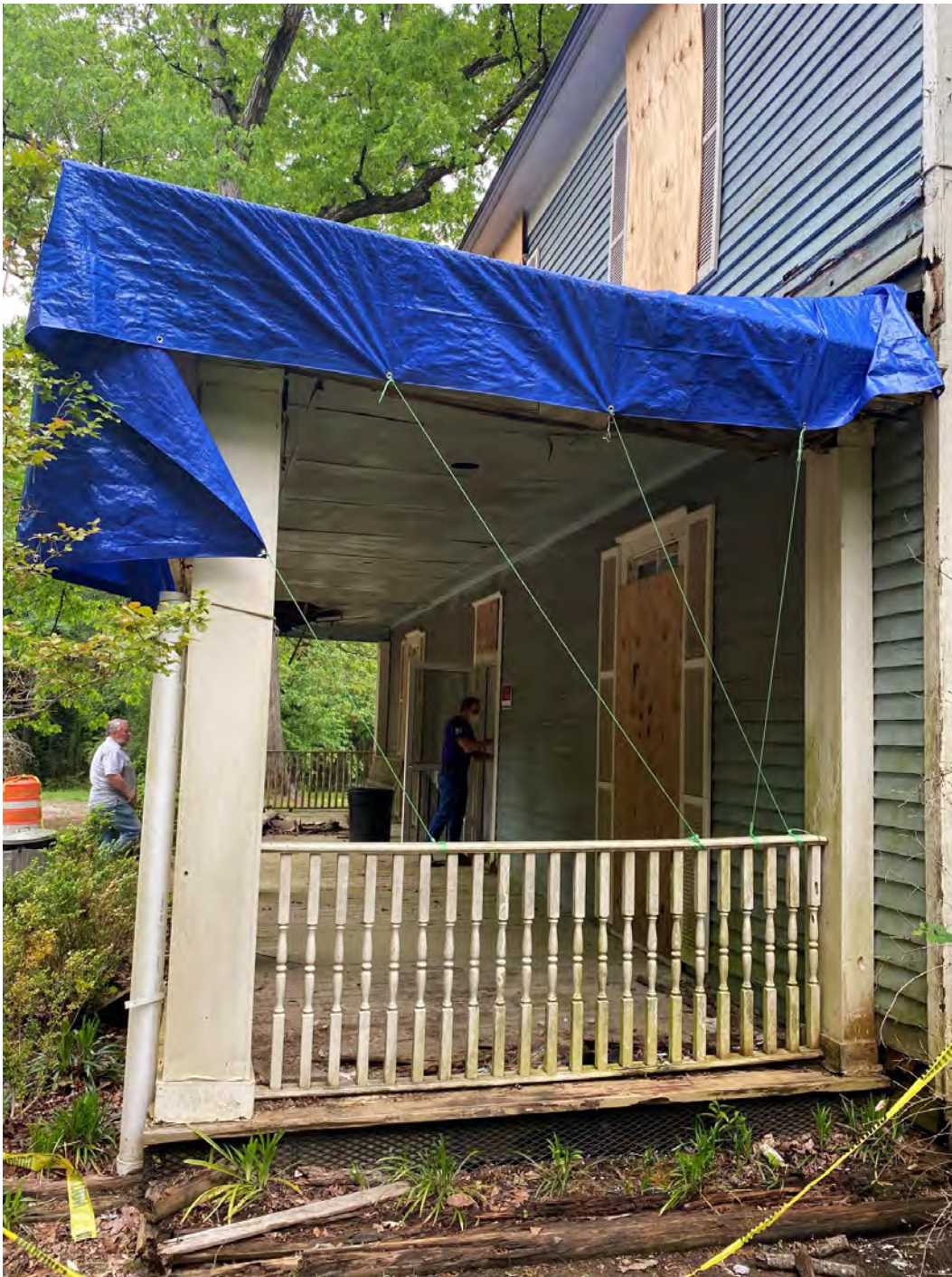
PHOTO 2: (View of North West Front Porch) - Porch in very poor condition.
