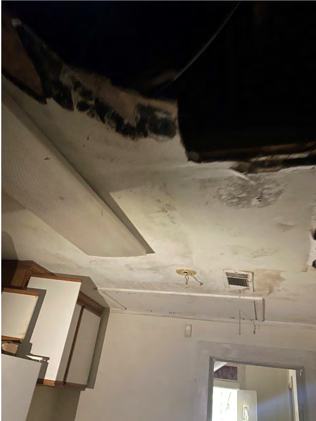
PHOTO 74: (View of Interior, Kitchen, Addition 1 & 2, hole in ceiling):
