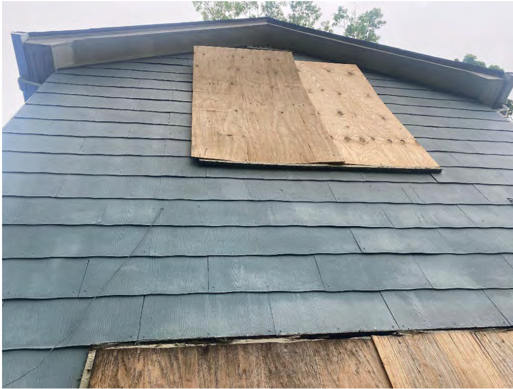
PHOTO 24: (View of Rear Façade, Addition 1): Possible Asbestos tile siding. - Windows boarded up, in fair condition. - Addition 1, in lesser quality craftsmanship than main structure.
