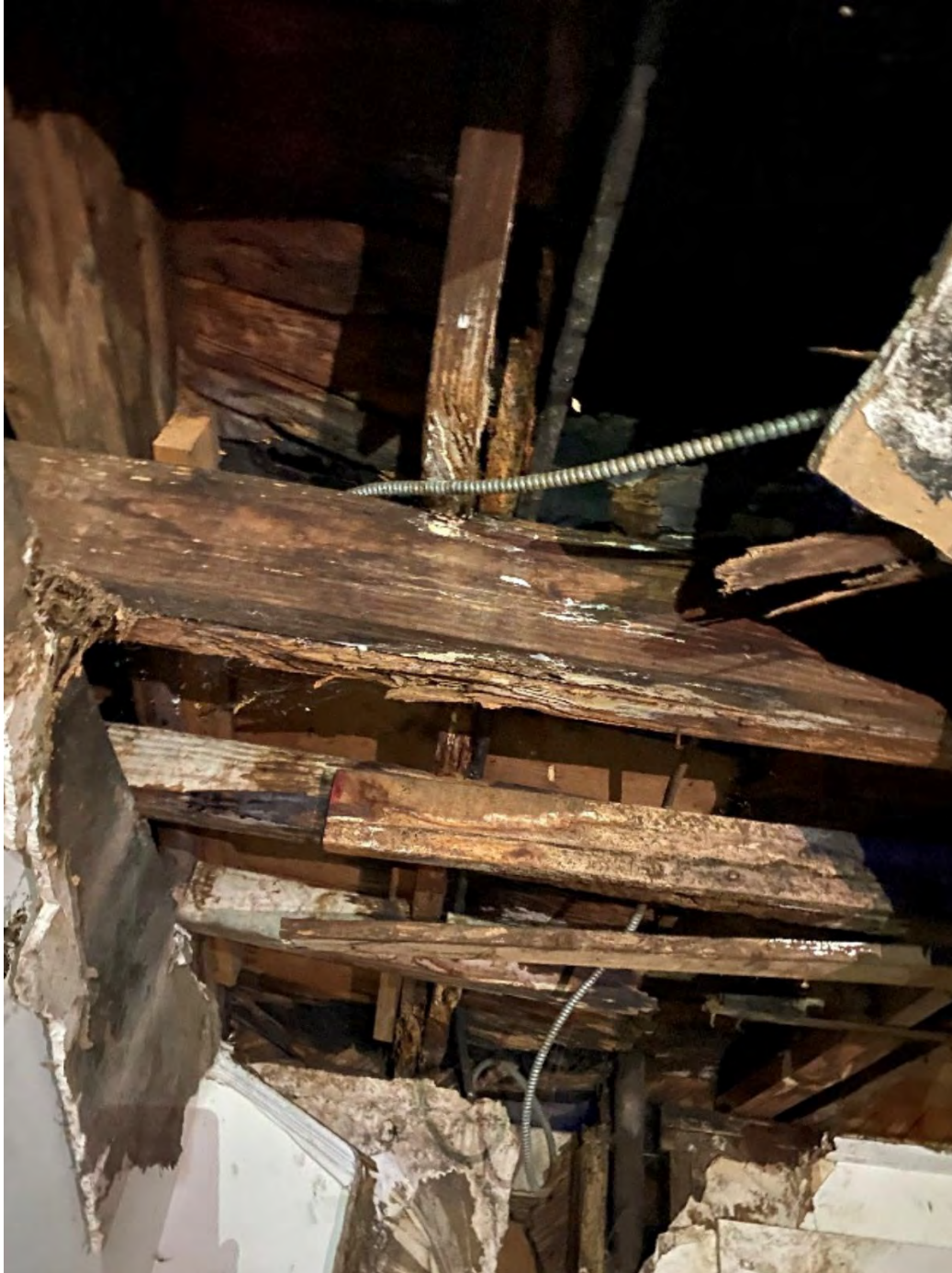
PHOTO 75: (View of Interior, Kitchen, Addition 1 & 2, hole in ceiling):
