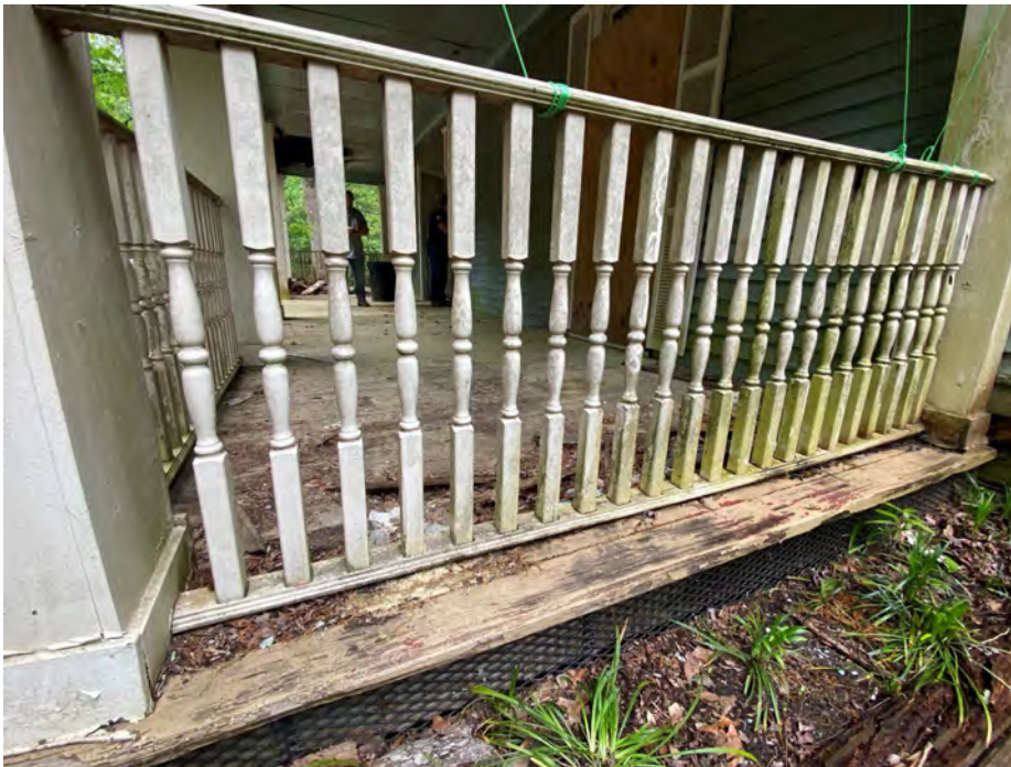
PHOTO 3 & 4: (View of North West Front Porch) - Porch in very poor condition.
