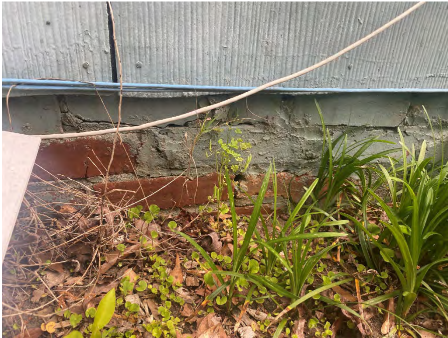
PHOTO 25: (View of Rear Façade, Addition 1): Brick Foundation.. - Foundation, no issues observed on exterior, floor uneven on inside rear.
