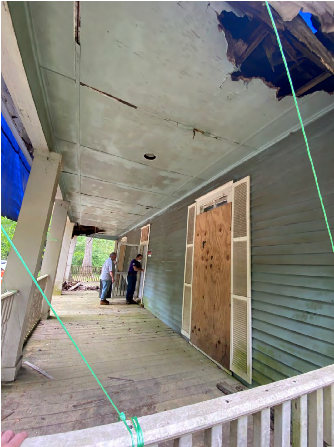
PHOTO 5: (View of North West Front Porch) - Porch in very poor condition.
