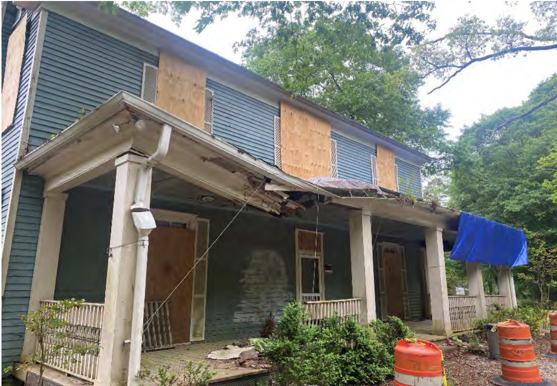
PHOTO 9: (View of North East Front Porch) - Porch is collapsing.
