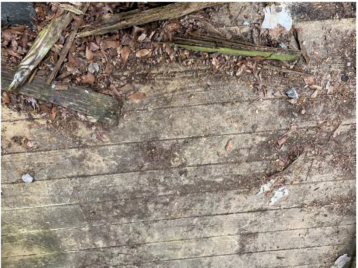
PHOTO 6, 7, & 8: (View of North West Front Porch) - Porch in very poor condition.
