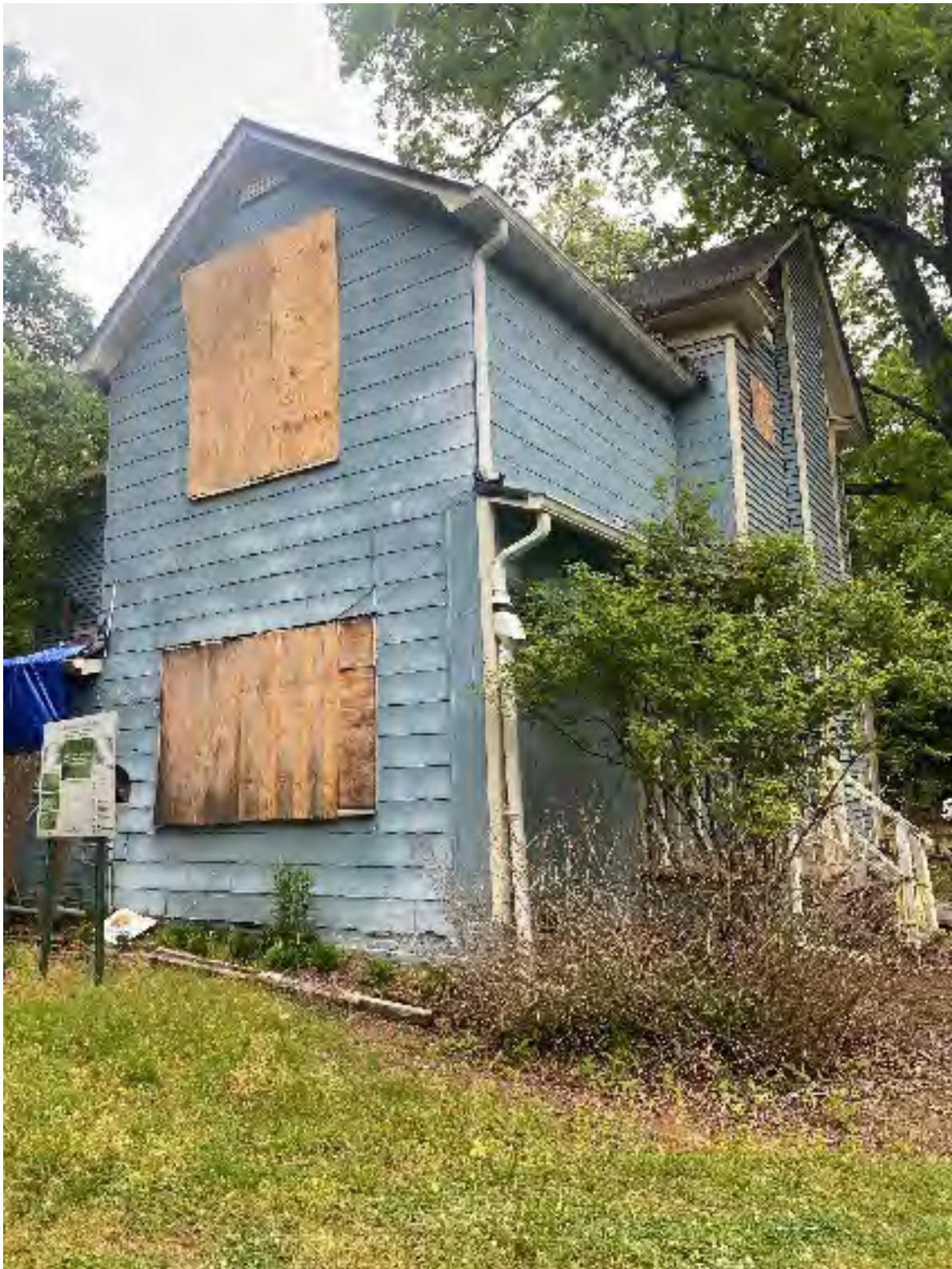
PHOTO 23: (View of Rear Façade, Addition 1): Possible Asbestos tile siding observed.
